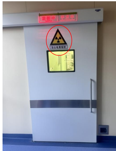
7号楼一楼DSA机房防护小门
